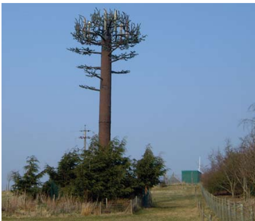
Telephone mast near Bassenthwaite Lake - Photo by Cumbria County Council
